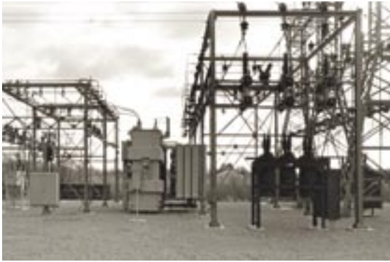
Trails Corner Substation prior to the addition in 1992.
