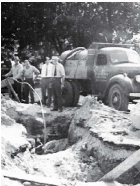
Early on, GU workers regularly made repairs and improvements to the city's water lines, as seen here in this 1950s photo.
